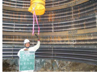
換気用送風機風量確認
